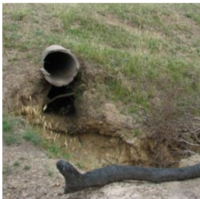
Plate 13 Dam failure around overflow pipe
