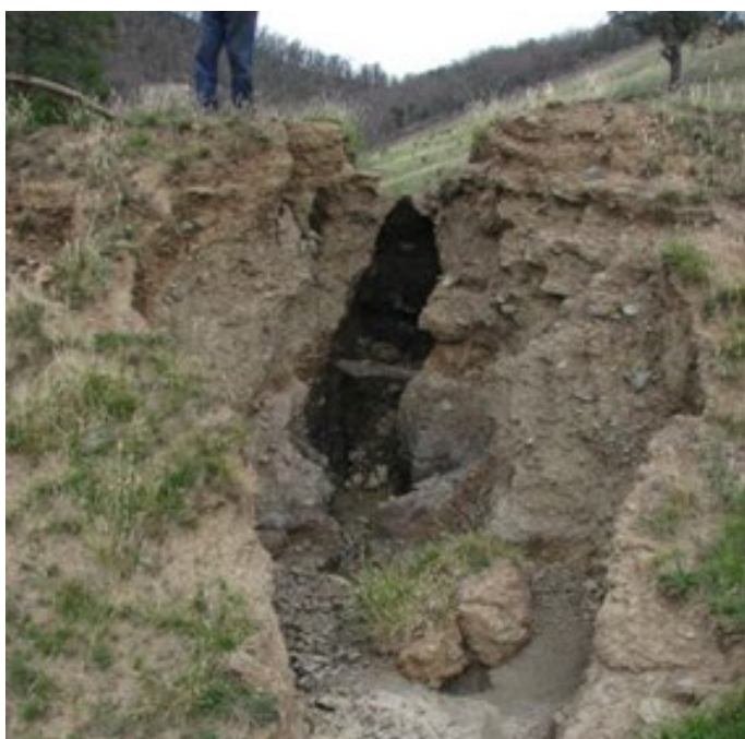
Plate 12 Dam embankment failure following the Kilmore East - Murrindindi bushfire
