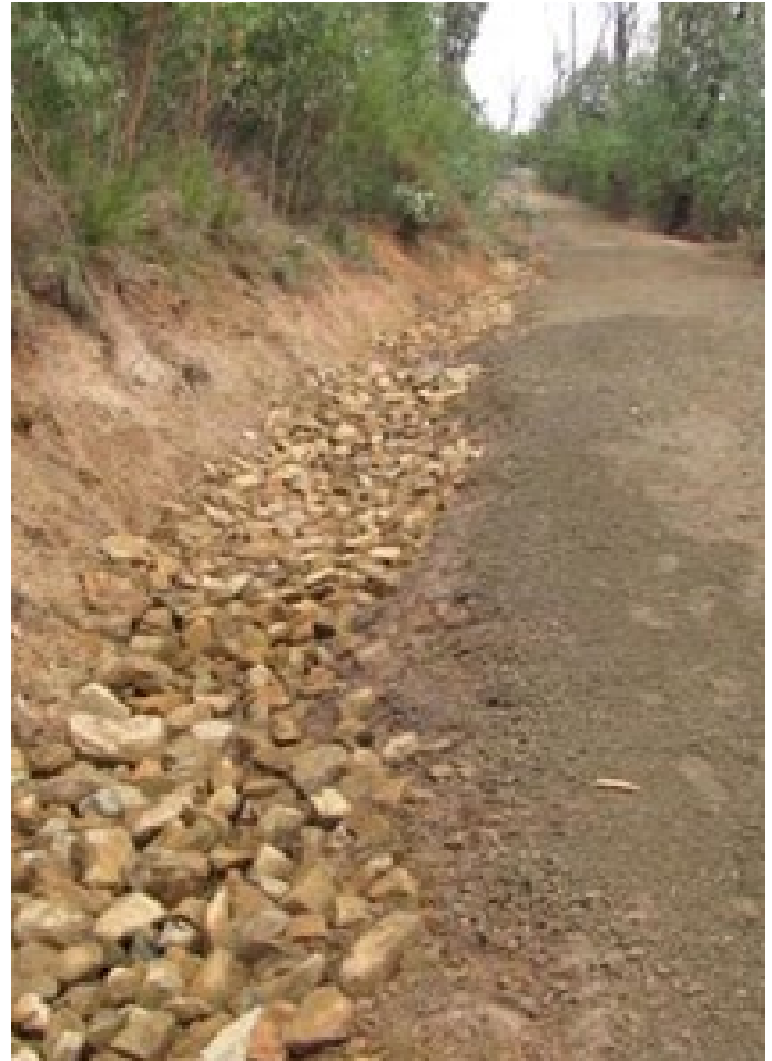
Plate 20 Armouring of roadside drainage channel
