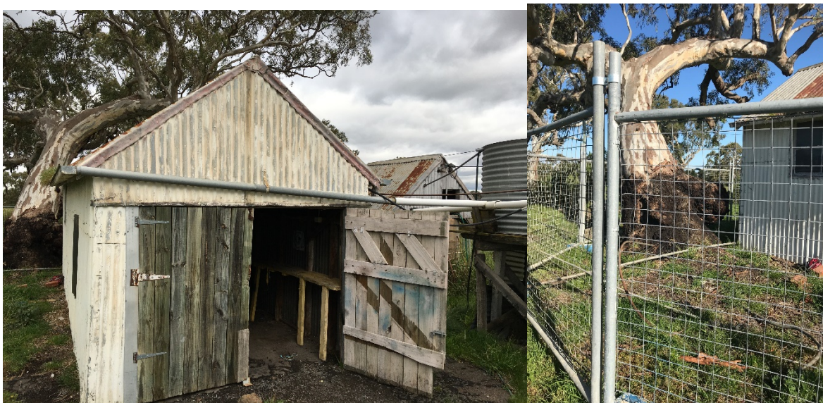
Figure 10 – South southwest to the structures at the southern corner of the weatherboard dwelling. 20 May 2020.
