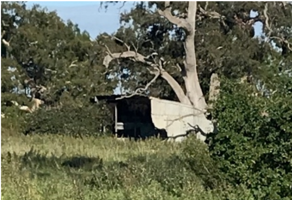
Figure 12 – Open-sided shed structure south southwest from the east side of the weatherboard dwelling. 11 May 2020
