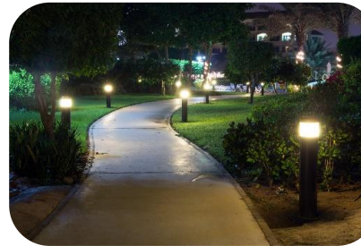
Example of lighting
