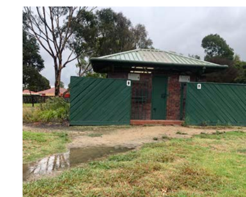
C No DDA access path to the public toilet & subject to flooding
