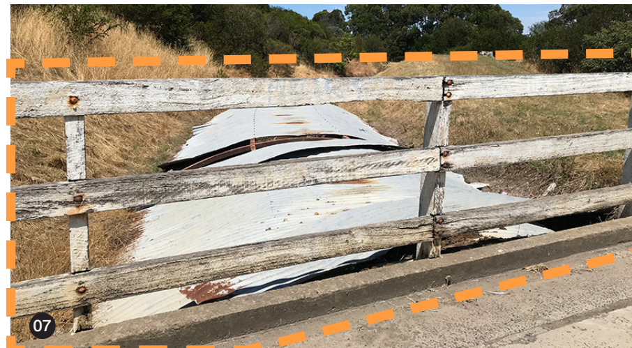
07 Example of dilapidated timber fencing at Evelyn Street
