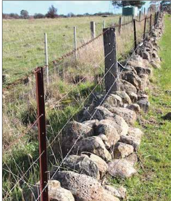
Image 31: William Bodycoat farm wall. Its height and construction are reasonably uniform, and the narrower base suggests it was not an original all-stone wall. Timber posts are reasonably uniform, and regularly spaced, although almost certainly replaced. Star pickets obviously inserted later. Such walls require closer physical investigation to determine whether originally composite, or modified later. (David Moloney, 2019)
