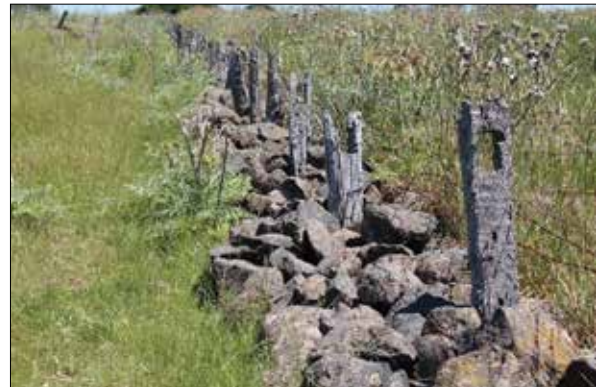
Images 34, 35: The composite wall in 2019 (left) has deteriorated since 2011 (right).
