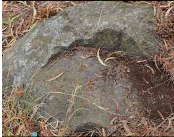
Image 27: Flatter slightly saucer-shaped stones often appear in Whittlesea walls, usually as a bedding or plinth ('coverband') for the copingstones (the top course). But in the wall above and elsewhere in Whittlesea they are also fitted into the wall, in the manner of traditional plugging. These naturally broke off the top of rock in outcrops as shown here, or could be easily knocked off, as water in fissures froze and cracked the stone. The same process would have applied for large stones, which split off along weathered natural fractures on outcrops, or could be easily prised apart. (David Moloney, 2019)
