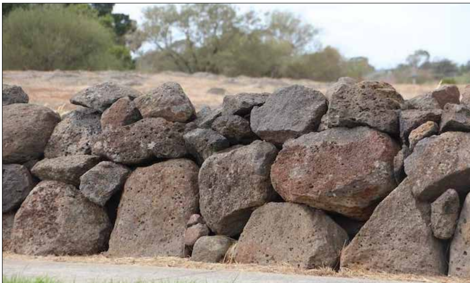
Image 106: The practical craftsmanship of this same Gardenia Road wall is more evident here. The difficult, oversize stones, which have likely been grubbed from the stony rises on the church reserve behind, have been carefully positioned and their split flat surfaces arranged to present a relatively smooth and battered wall face. It appears to have been repaired, but its original form was that shown in the 1885 photograph (Image 113) of the nearby cemetery wall: higher and with coping stones intact. (David Moloney, 2019)
