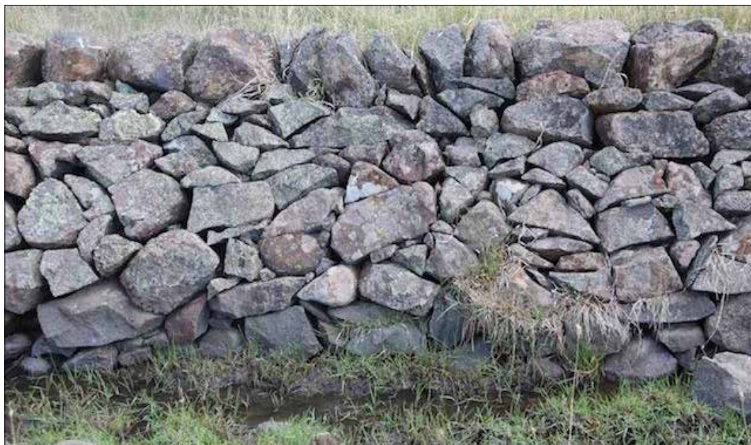
Image 139: Wall face of part of the remarkable stream diversion retaining wall between Lehmanns and Bridge Inn Road, built by Gottlob Ernst Schultz and his sons. The height of this part rises to 1.3 metres. There is a stone apron under the channel in front; the coping stones are at the level of the ground on the other side of the wall. (David Moloney, 2013)
