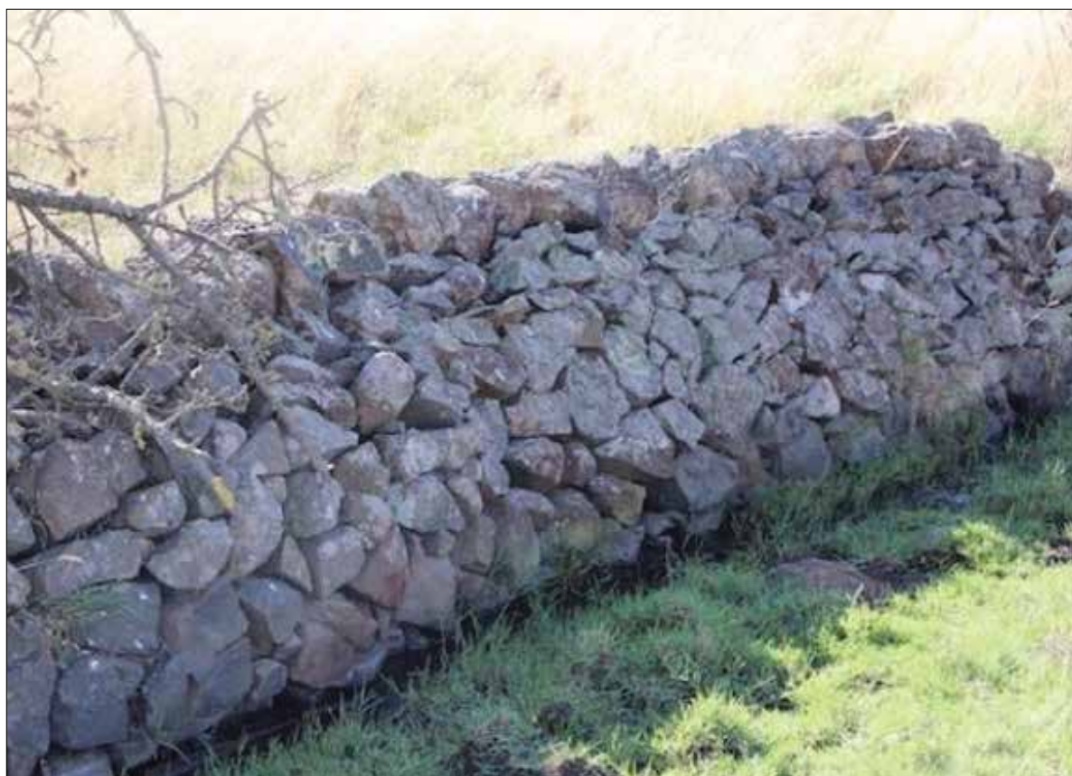
Image 63: Former retaining wall built to channel and drain water on former Schultz property, south side of Bridge Inn Road. Fragments of the stone base of the channel is visible. It is beautifully constructed, mainly with quarried angular stone in this section, with round field-stone as coping. (David Moloney, 2013)
