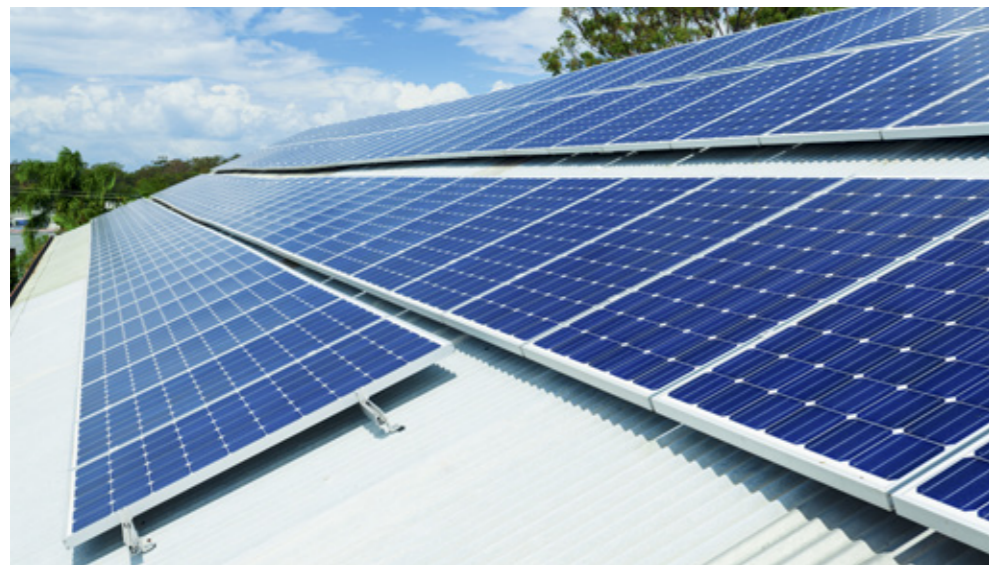
ABOVE The solar array on the roof of Thomastown Library.
