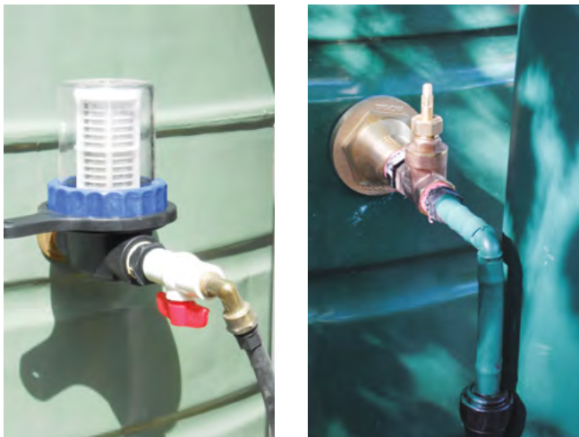
Figure 8 Low-flow control through ball valve and inline filter (source: University of Melbourne)
