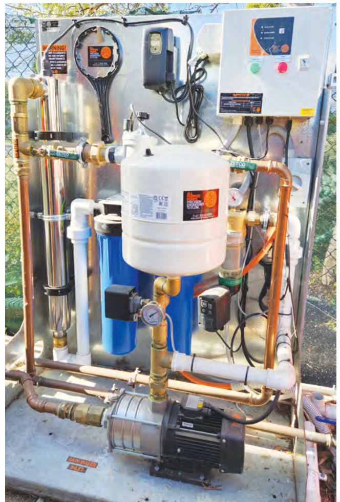
Figure 14 Commercial-scale reclaimed rainwater treatment, Houston Street Depot, Epping
