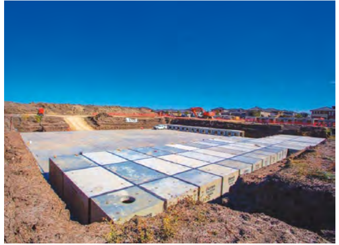
Figure 15 Underground storage of the Mosaic stormwater harvesting scheme in Lalor
