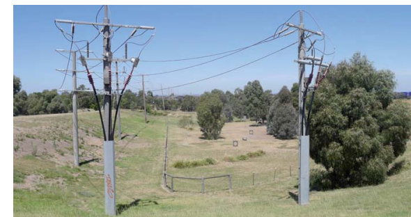
Photo 2: Existing High Voltage Transmission Lines
