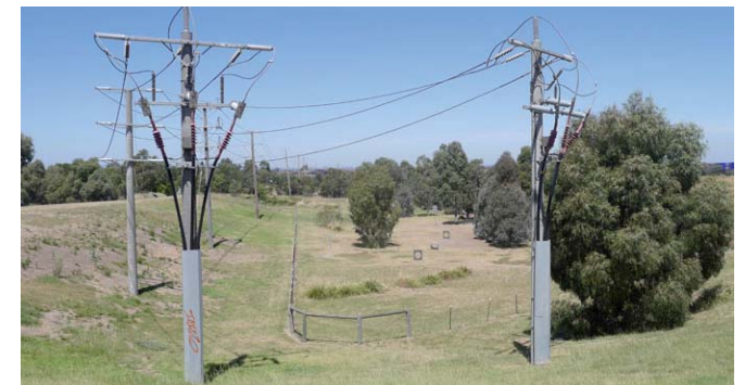
Photo 2: Existing High Voltage Transmission Lines
