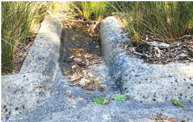
Figure 46 Sediment forebay at kerb entry (roadside biofilter in Fernhill Road, Mount Evelyn)
