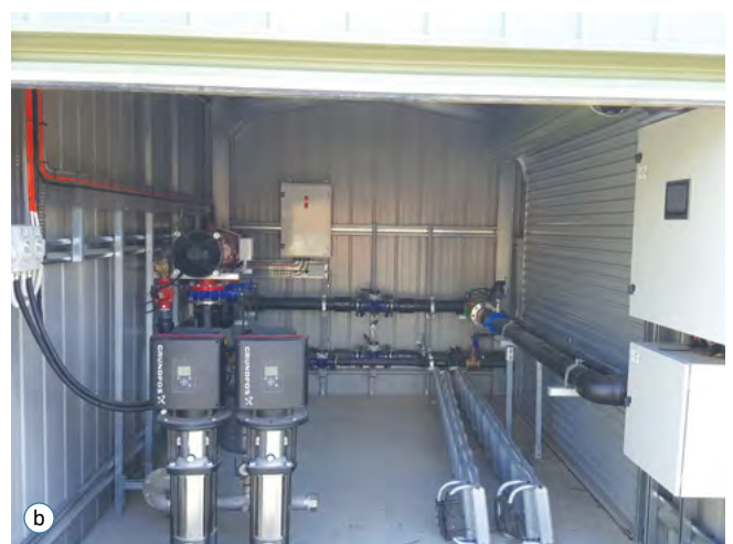
Figure 17 Different types of instrumentation housing: a) Enclosure style at Laurimar Recreation Reserve, Doreen b) Pump room style at Pinks Reserve, Kilsyth
