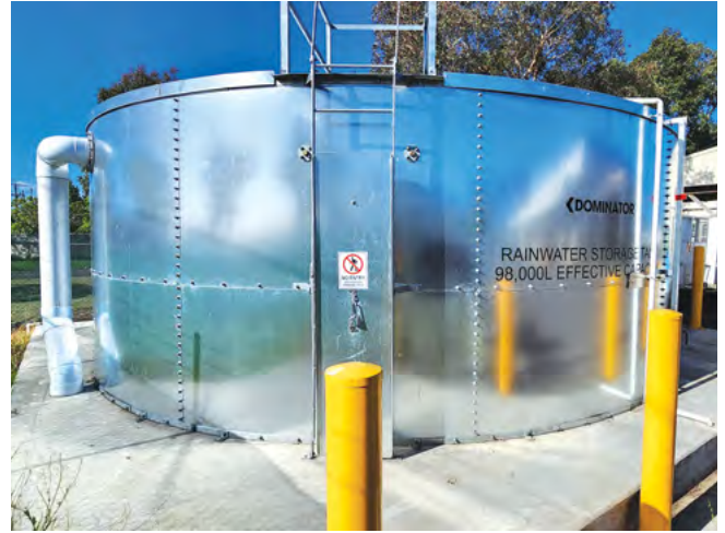
Figure 7 Rainwater tank at Houston Street Depot, Epping
