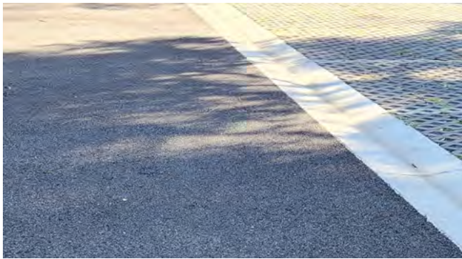
Figure 29 Open graded asphalt wearing course on School Road car park, Menzies Creek
