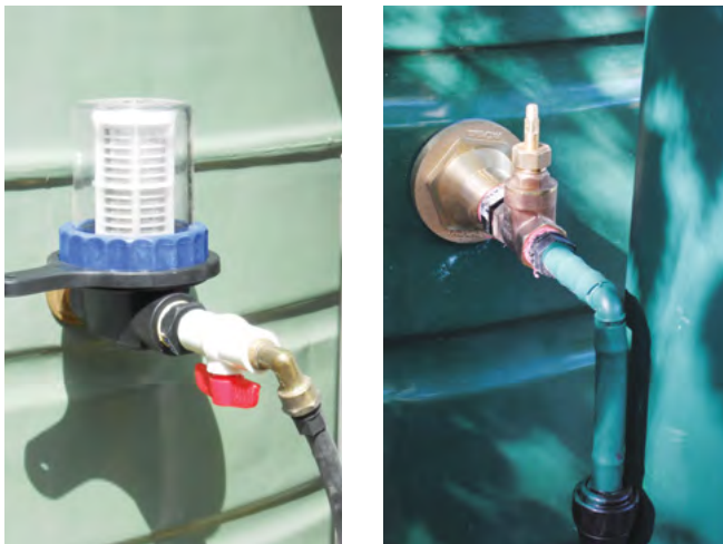
Figure 8 Low-flow control through ball valve and inline filter (source: University of Melbourne)
