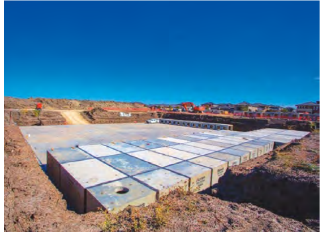
Figure 15 Underground storage of the Mosaic stormwater harvesting scheme in Lalor
